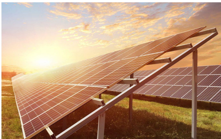
Figure 8: Bangladesh Largest Solar Power Plant Connected to National Grid
